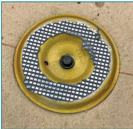
Figure 13 – The top of an induction-welded fastener plate showing membrane delamination (cap to core separation).
